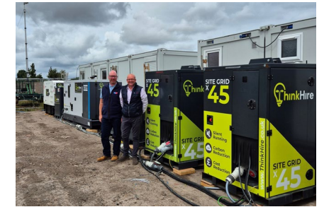
Hybrid Generators – Moss Nook
